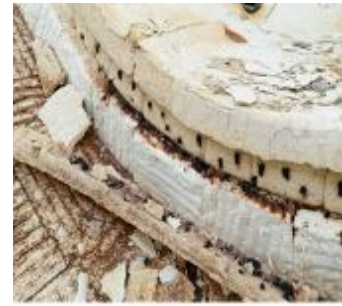
Gambar 3. Adanya serpihan material castable refractory
